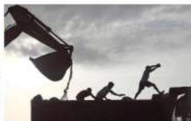
Workers use machinery at a canal roof project construction site in Mumbai.
